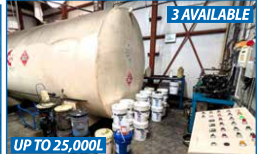
PARTIAL VIEW OF DTE BULK STORAGE TANKS
