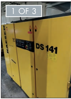
KAESER 100 HP AIR COMPRESSOR
