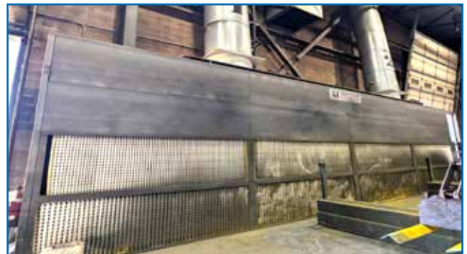
UNITED INDUSTRIAL PAINTING EXHAUST / FILTRATION UNIT
