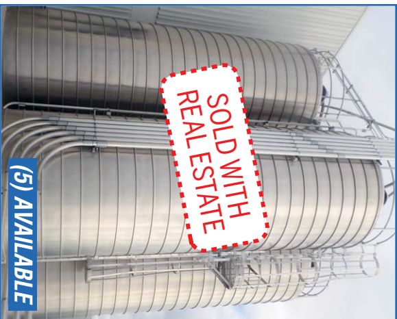
PARTIAL VIEW OF S/S SILOS
