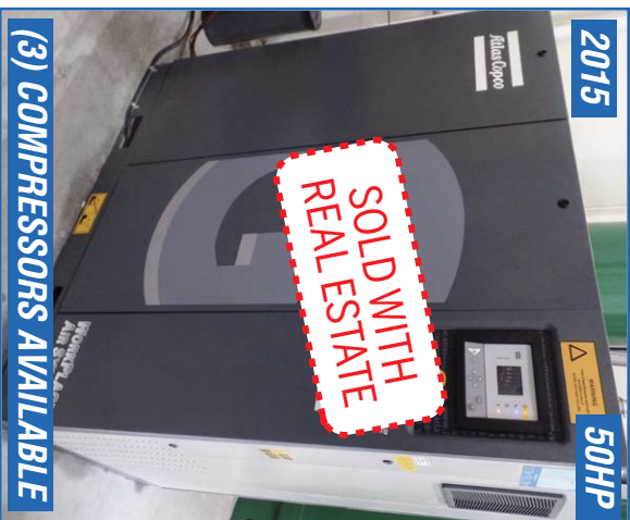
ATLAS COPCO GA37VSD FF COMPRESSOR
