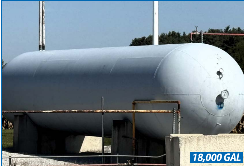
TRINITY STEEL PROPANE STORAGE TANK W/ RANSOME RH200E VAPORIZER
