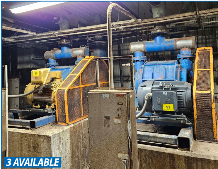
PARTIAL VIEW OF NASH VACUUM PUMPS
