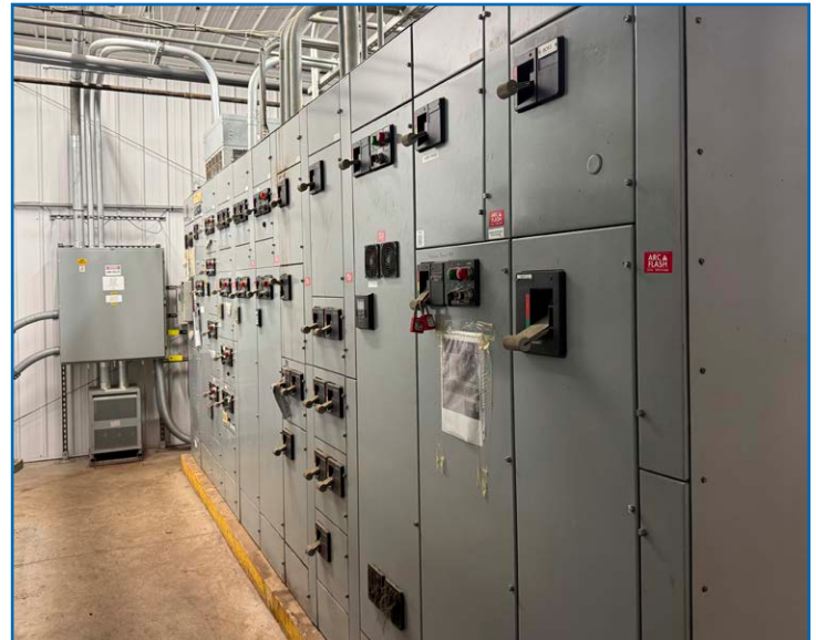
PARTIAL VIEW OF MCC'S, TRANSFORMERS, ELECTRICAL
