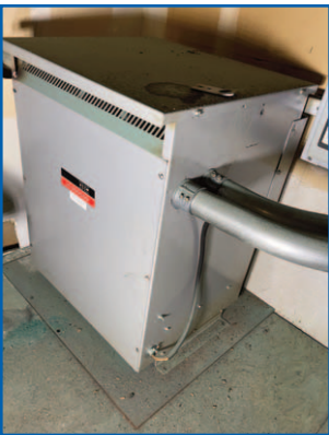
LARGE QTY OF TRANSFORMERS AND ELECTRICAL WIRE
