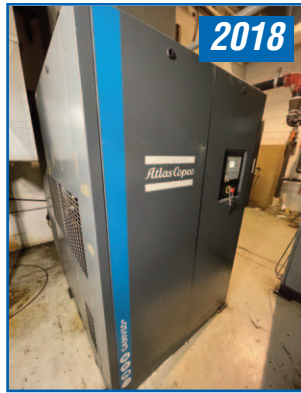
ATLAS COPCO GA90VSD AIR COMPRESSOR
