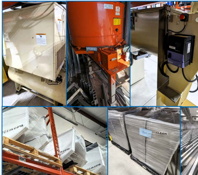
PARTIAL VIEW OF PLANT SUPPORT EQUIPMENT
